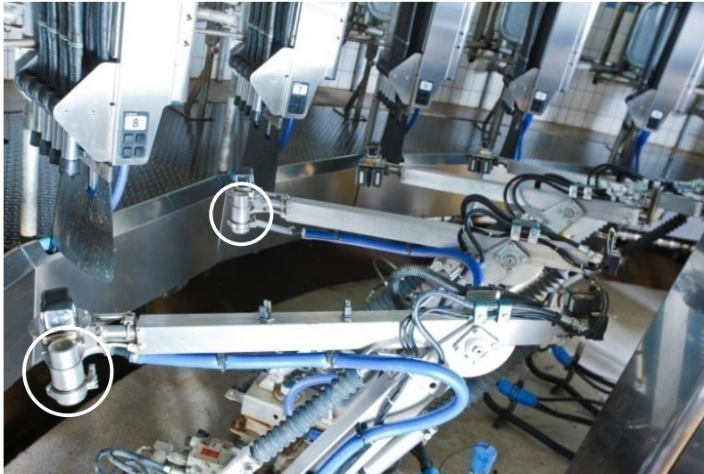
Figure 2.3: Robotic devices; installation of two teat preparation modules (TPM, in foreground) with fixed cleaning cups (circled) and two automatic cup attachers (ACA, in the background; www.DeLaval.com )
