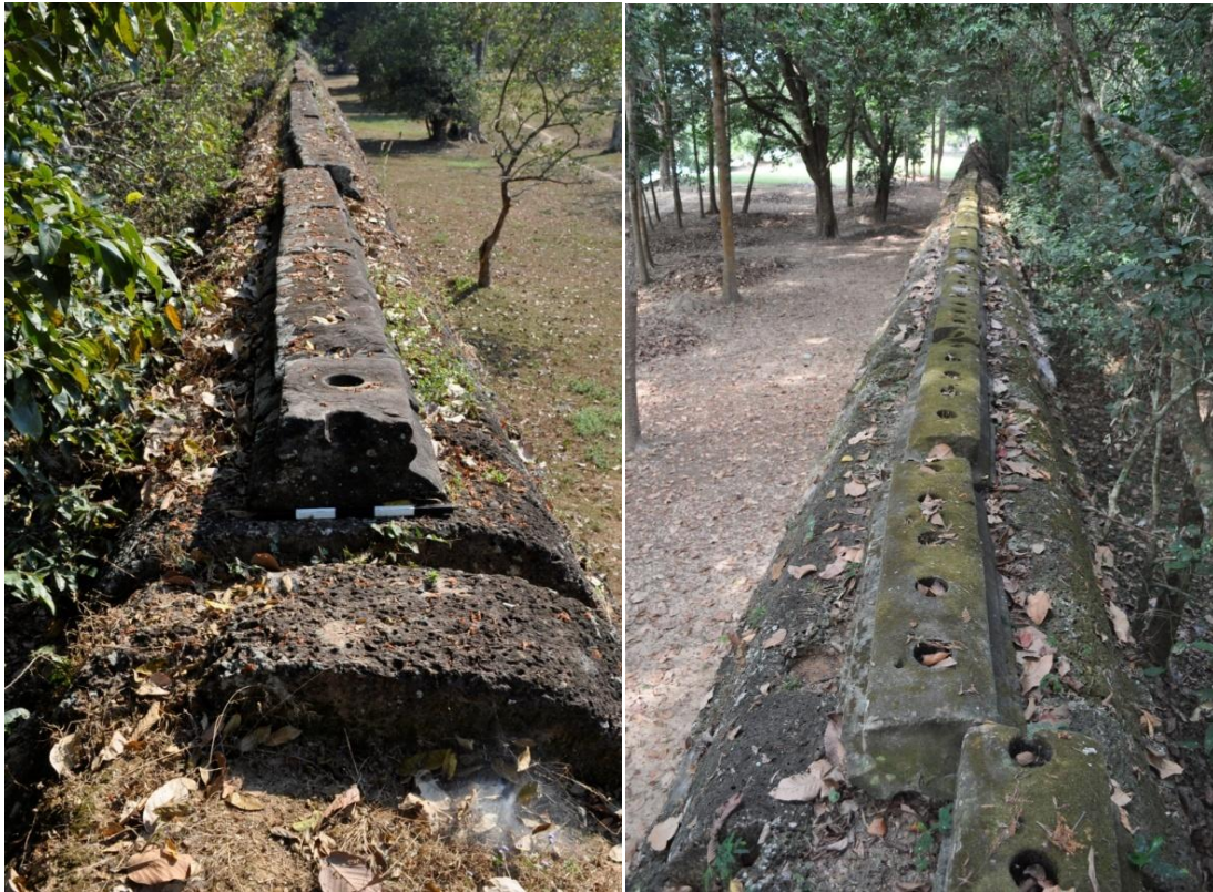
Figure 6.5 - Coping stones along the top of the West wall – Note the elongated shape.
