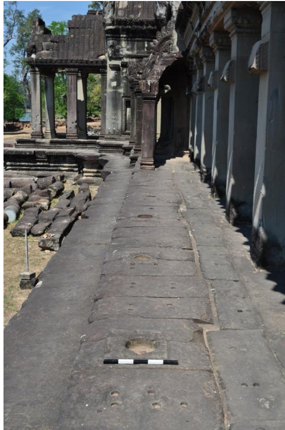
Figure 6.2 - West gopura, exterior, facing South – Note the postholes for the verandah columns (foreground), the sheared cross beams of the verandah (right), the missing stones of the porch roof (background, left) and the original verandah column and corbel vaulted roof in situ (background, centre)
