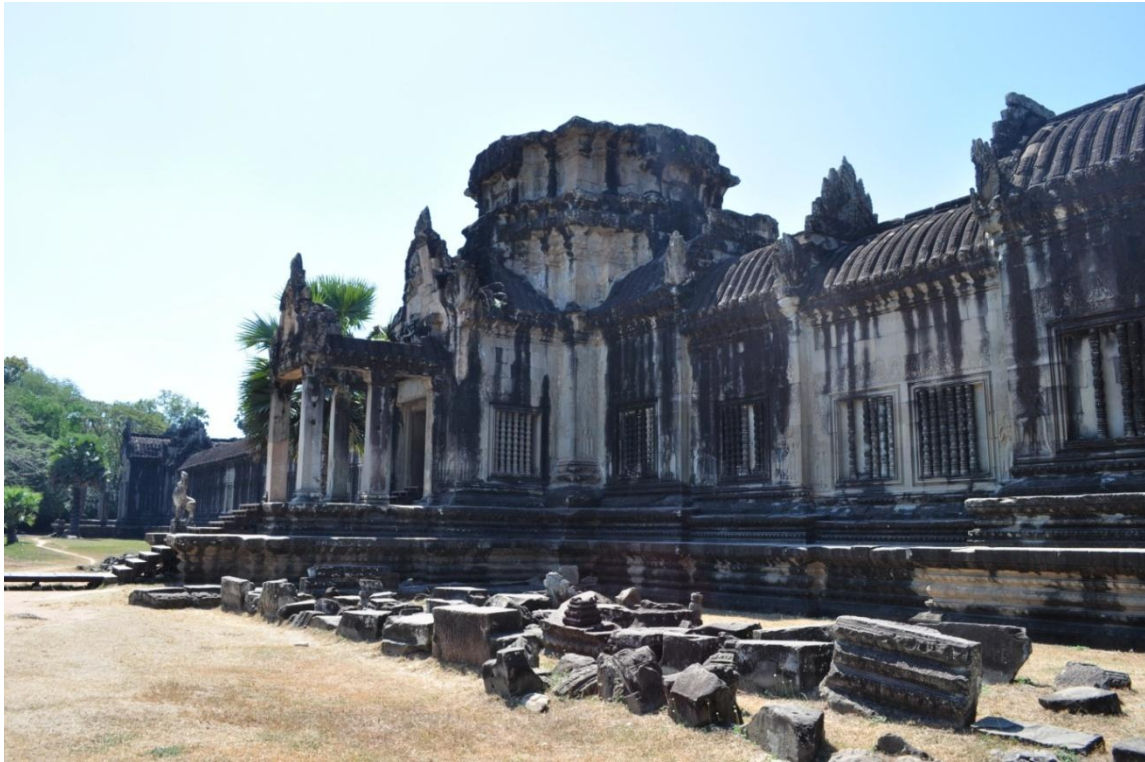
Figure 6.4 – West gopura, interior – Note the dislodged pieces of sandstone
