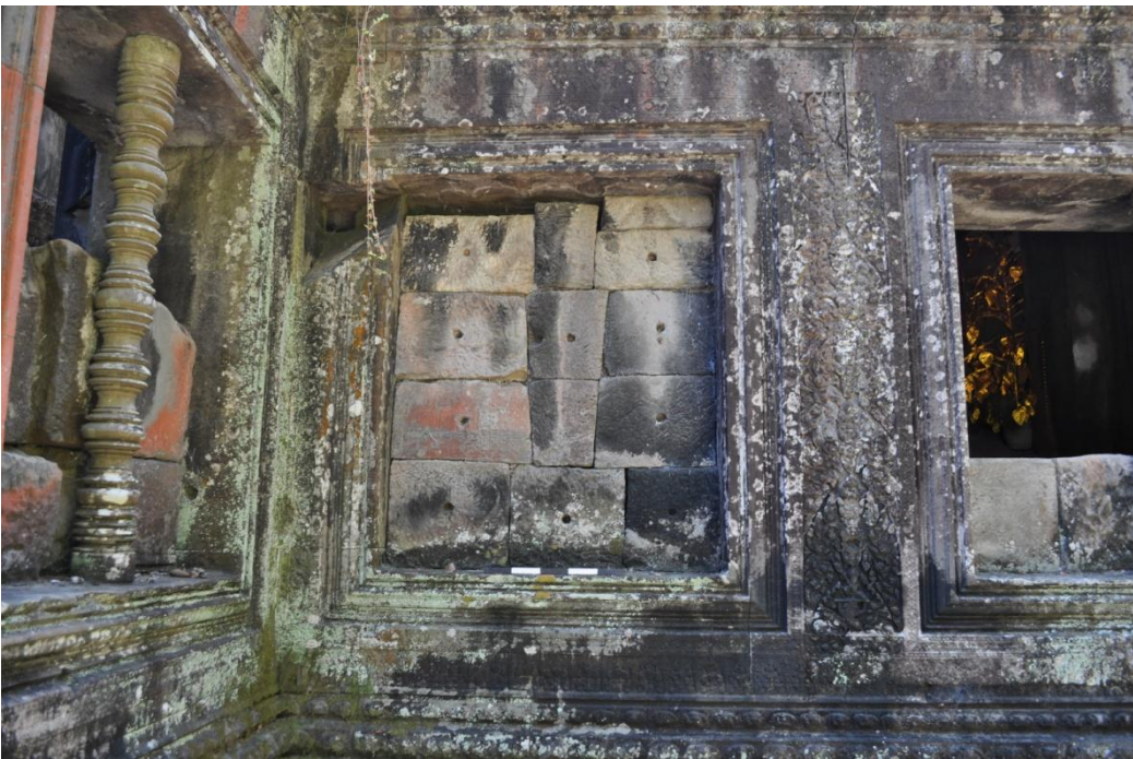
Figure 4.31 - The difference in block work between a false window (above) and real window with blocked up infill (below); South gopura, interior.
