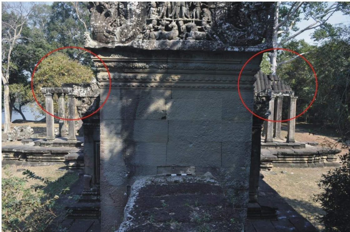
Figure 6.3 - North gopura, facing East - Note the missing stone pieces from the porch roofs and the architraves.
