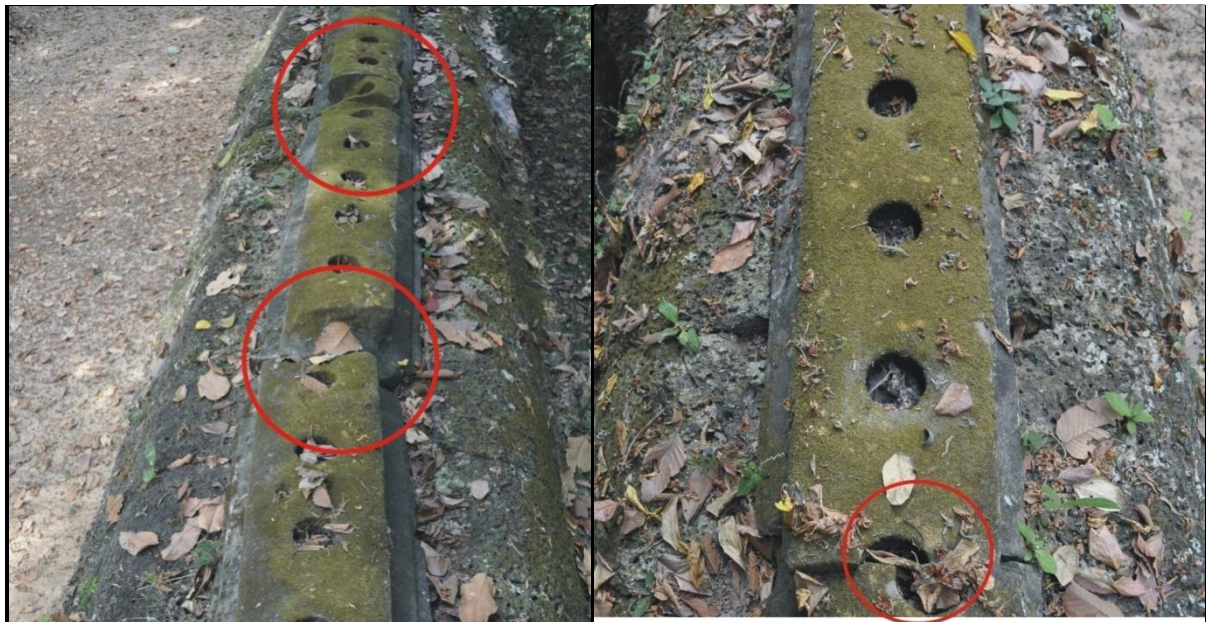
Figure 6.8 – Coping stones on the West wall - Note the breaks and broken ends.
