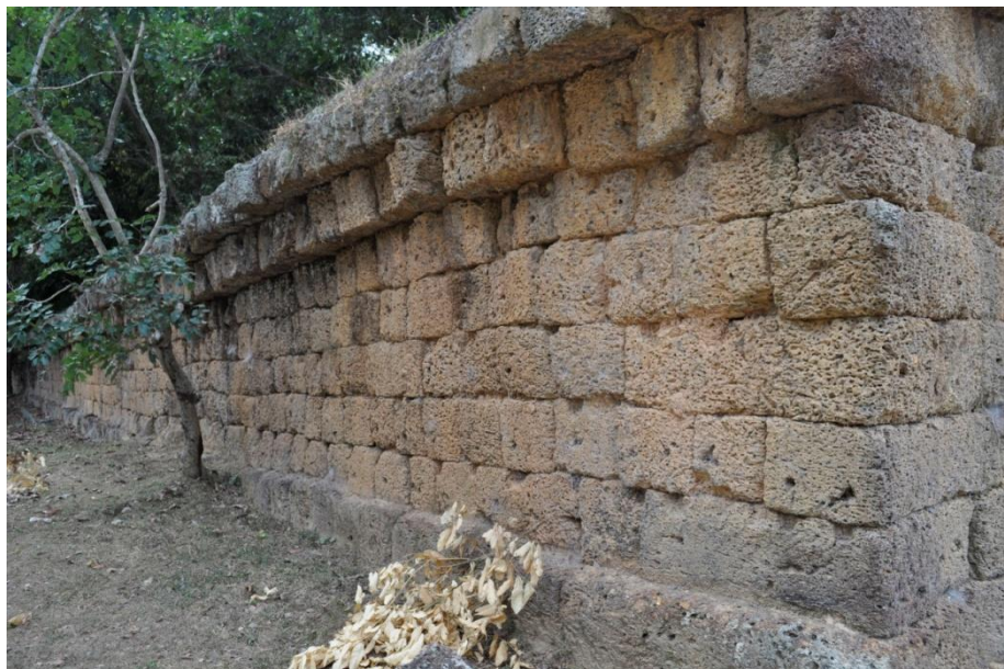
Figure 4.7 – Indentations, Northeast corner, exterior – Note their presence at all heights of the wall
