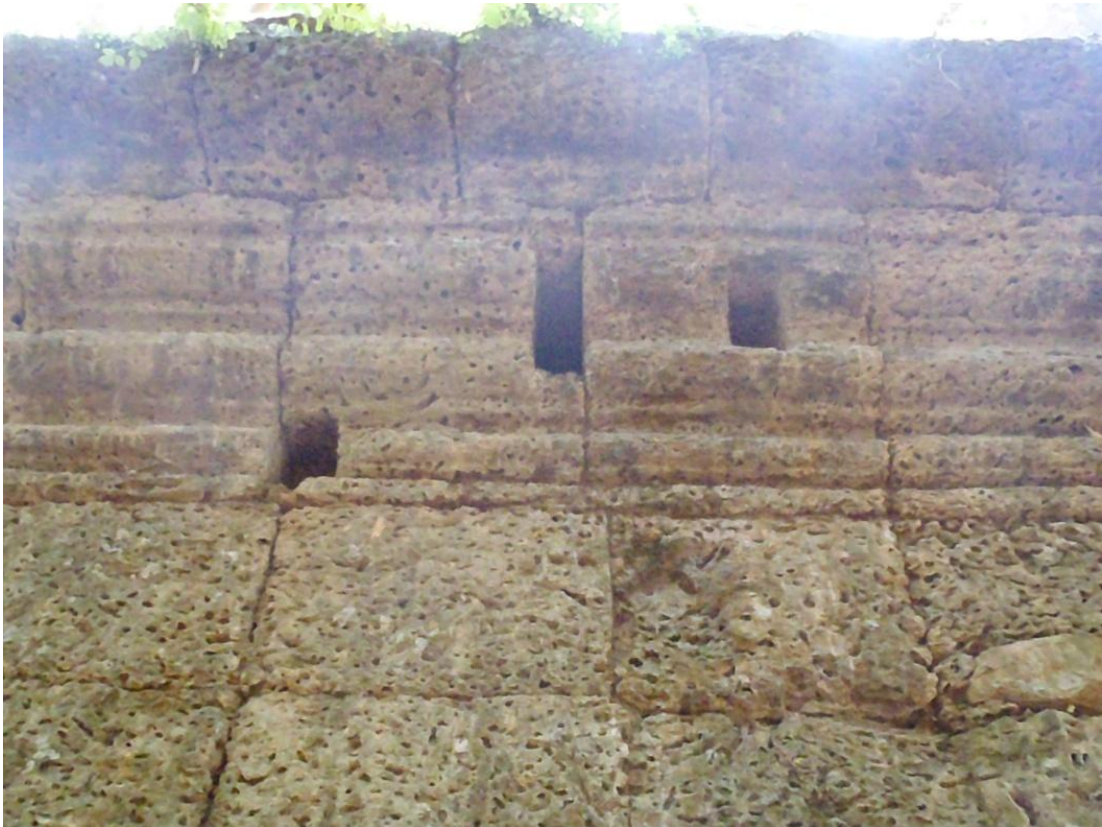
Figure 5.9 - A cluster of postholes: South wall, West side, near the South gopura.
