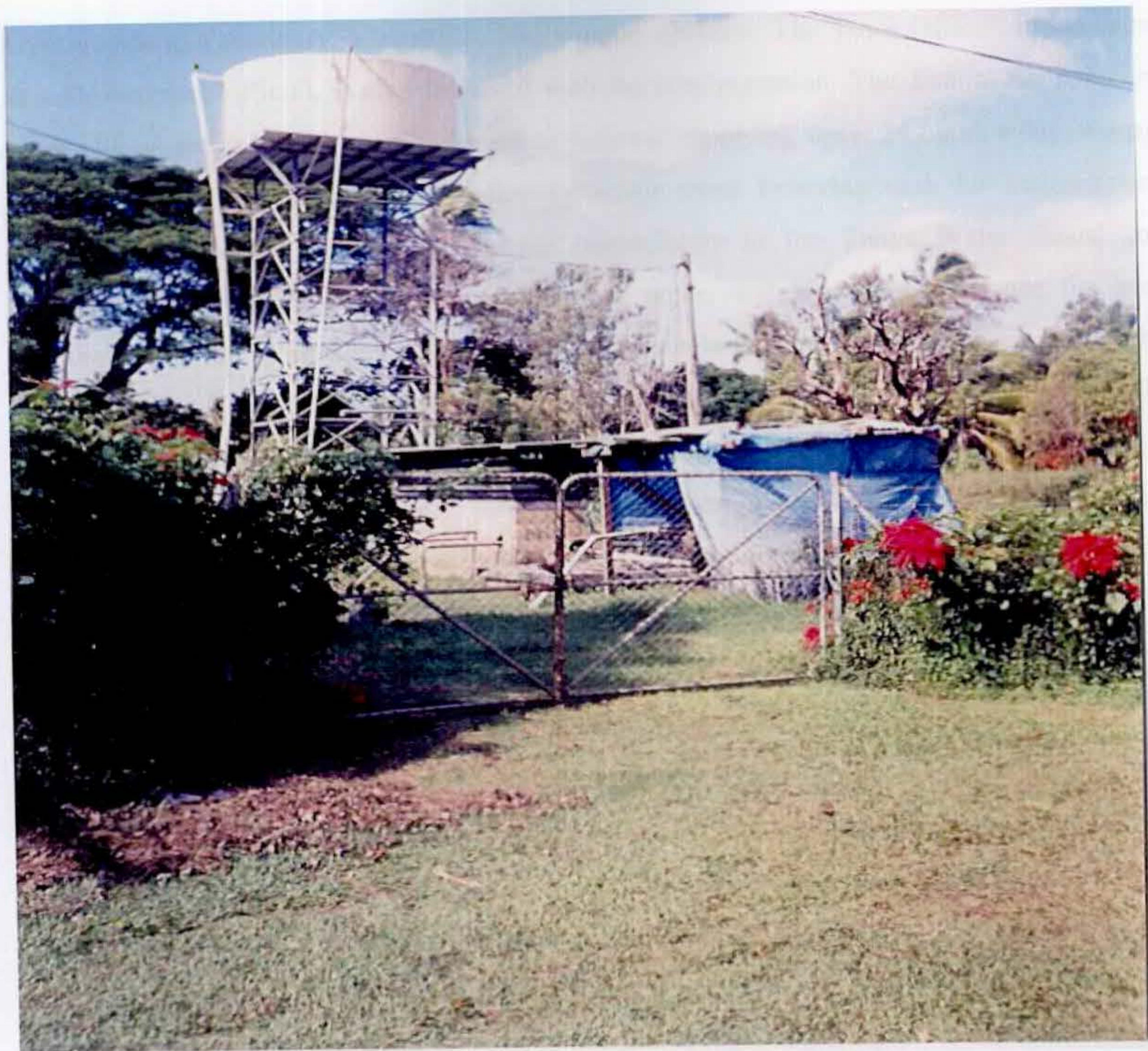
Figure 5.9 Water reservoir and water pump.
