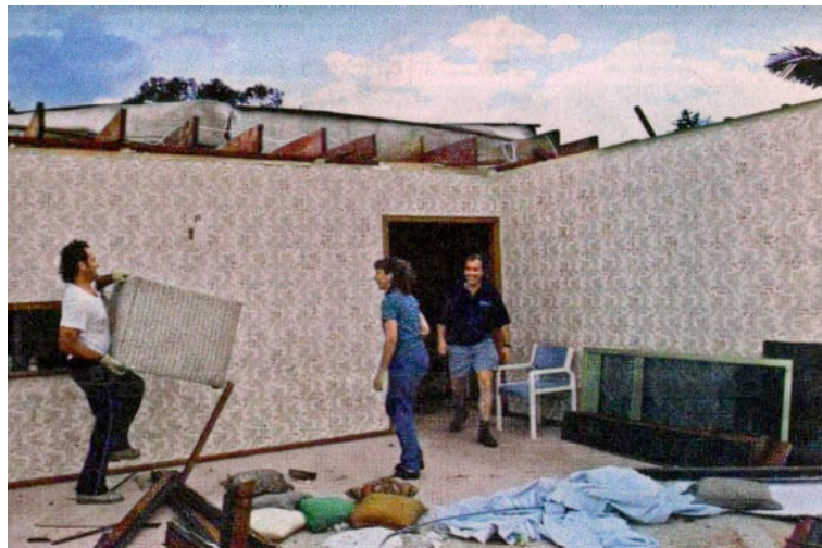
Plate 4.1 House damaged by storms
