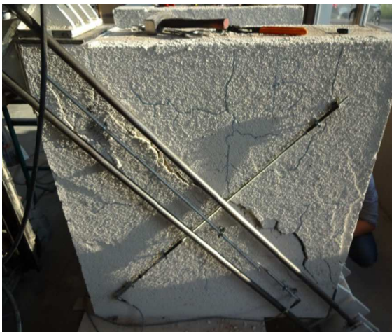
Fig. 8 Detail of the failure mode (panel reinforced with mortar Type RO)
