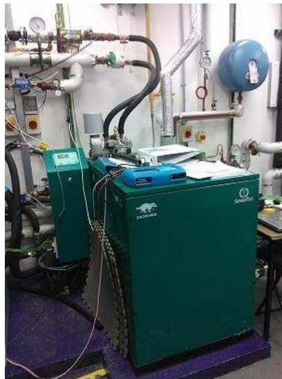
Figure 5.14 The Baxi SenerTech Dach mCHP unit installed in the Energy Laboratory
