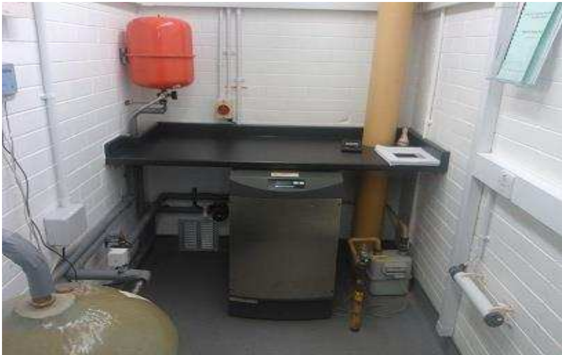
Figure 5.2 The Whispergen 1 kWe Stirling based mCHP installed in the Energy Lab
