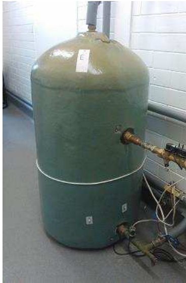
a) 150 L insulated hot water storage tank
