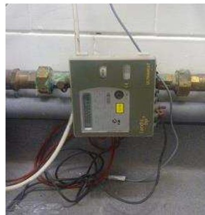
e) Heat meters measure and record the thermal energy supplied for both space heating and water tank.
