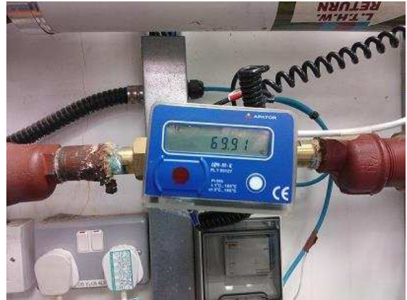
b) The Apator heat meter installed in the hydronic circuit
