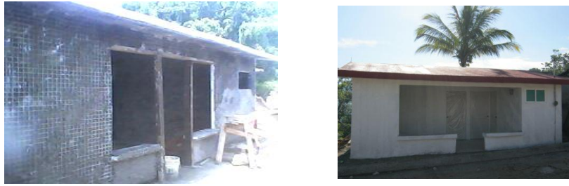
Figure 4 Mortar layer on 3D-LPs walls and figure 5 housing finished. Photo W Panel Company, 2013.
