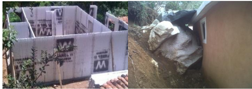
Figure 2 and 3 The 3D-LPs construction system used to build houses. Photos Credits: 1 and 2 from W Panel Company; Photo 3 Convintec Mexico
