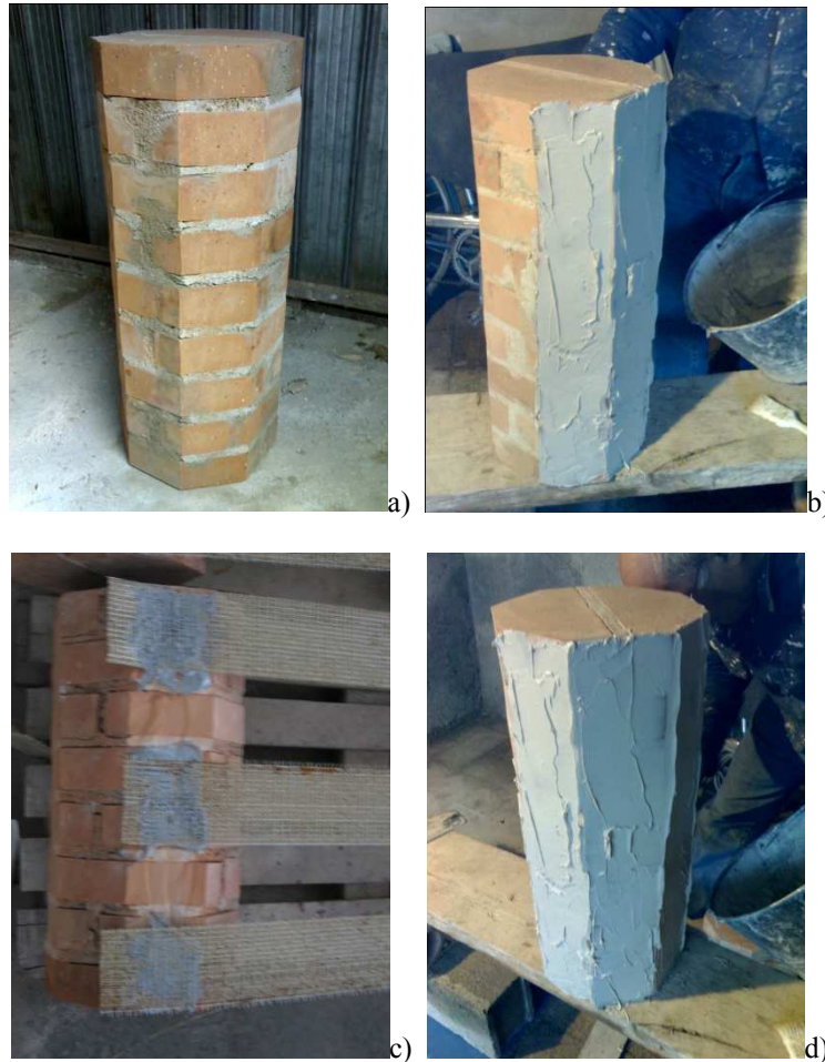
Figure 3. (a) Cleaning of the column surfaces; (b) Application of a first layer of matrix; (c) Application of a unidirectional SRP sheet; (d) Application of a second layer of epoxy resin or cementitious mortar.
