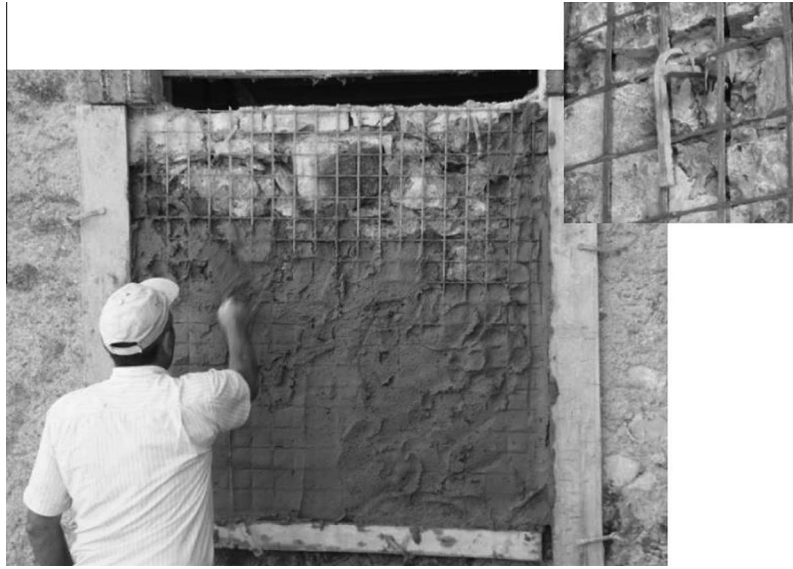
Fig. 5. Application of mortar jacketing and detail of connection between anchors and GFRP grid.
