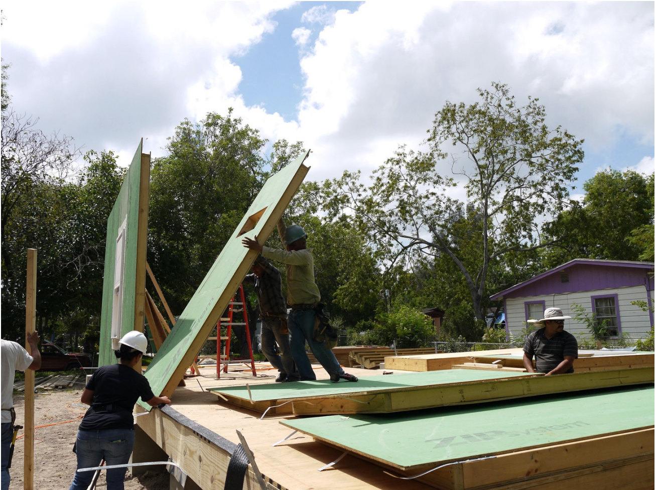
Figure 1. Photograph showing the installation of SIPs in the core of a RAPIDO prototype home. Source: bcWORKSHOP (2016).
