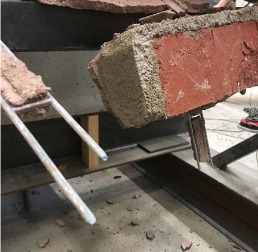
Figure B3_W1_1 Masonry reinforcement bars that failed in tension.
