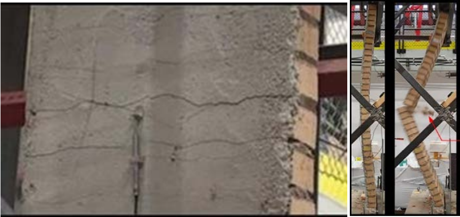
Figure B1_W5_3 Cracks at mid-height of the wall just before failure (left); Collapse of the wall (right).
