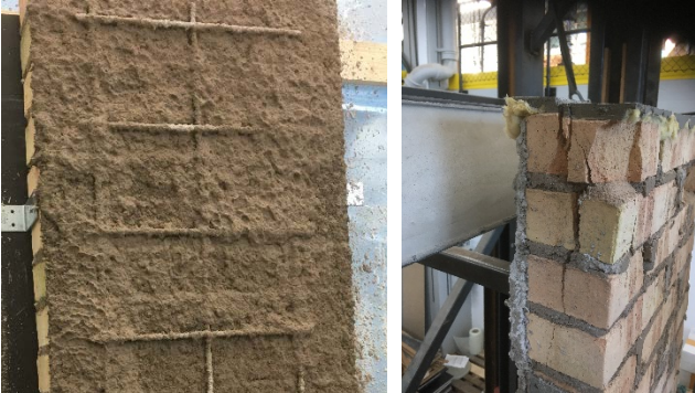
Figure B1_W1_1 Application of the first render layer, CS IV, thickness 3 – 8 mm (left); Failure at the upper loading plate (right).
