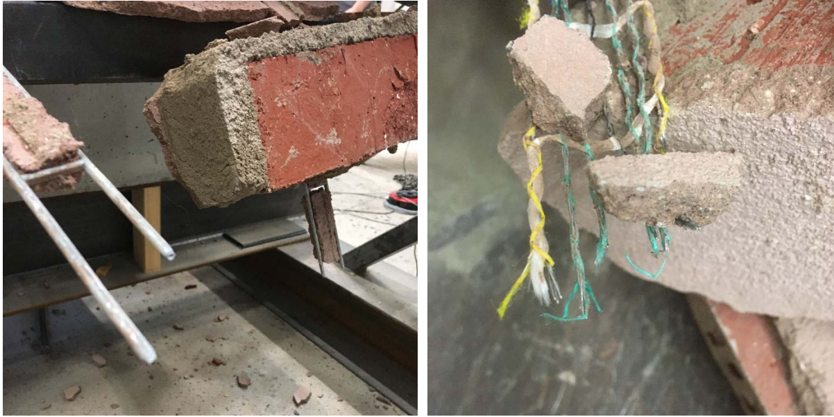
Figure 3.4 Tensile failure of strengthening, followed by collapse of the brick walls. Masonry reinforcement (left), high strength steel wire strip (right).
