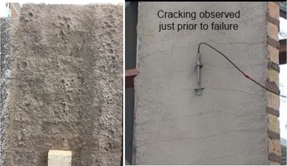
Figure B1_W4_1 Brick wall strengthened with strips of high strength steel wire, before application of the second layer of strengthening render (left); Crack pattern just before failure (right).
