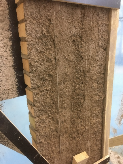
Figure B1_W2_1 Brick wall with masonry reinforcement (bistål), before application of the second strengthening render layer.
