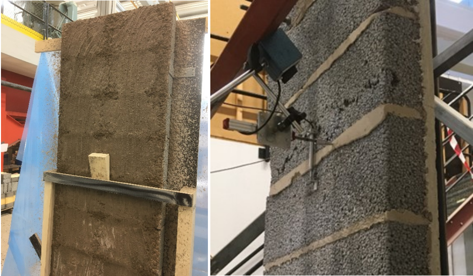
Figure LWA1_W2_1 Masonry reinforcement (left); Flexural compressive failure at mid-height of the wall (right).
