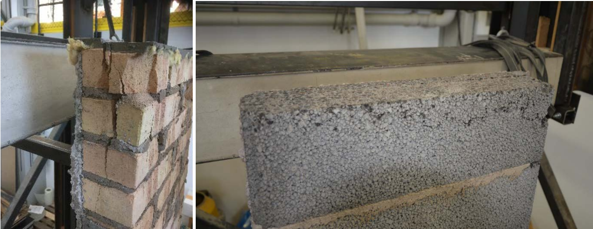
Figure 3.6 Crushing and splitting of masonry in the vicinity of the upper support.
