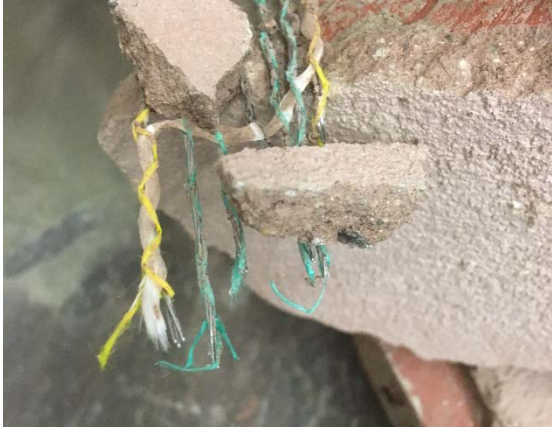
Figure B3_W3_1 High strength steel wires that failed in tension.
