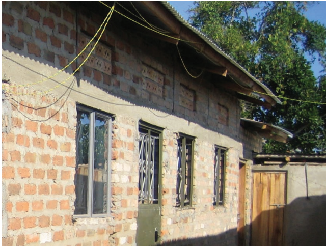
Figure 2. Permanent ventilators on windows and doors
