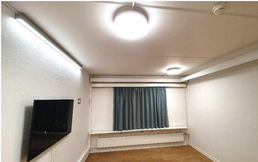
FIGURE 6. Picture of the room with existing electrical lighting (Dobos, 2020)
