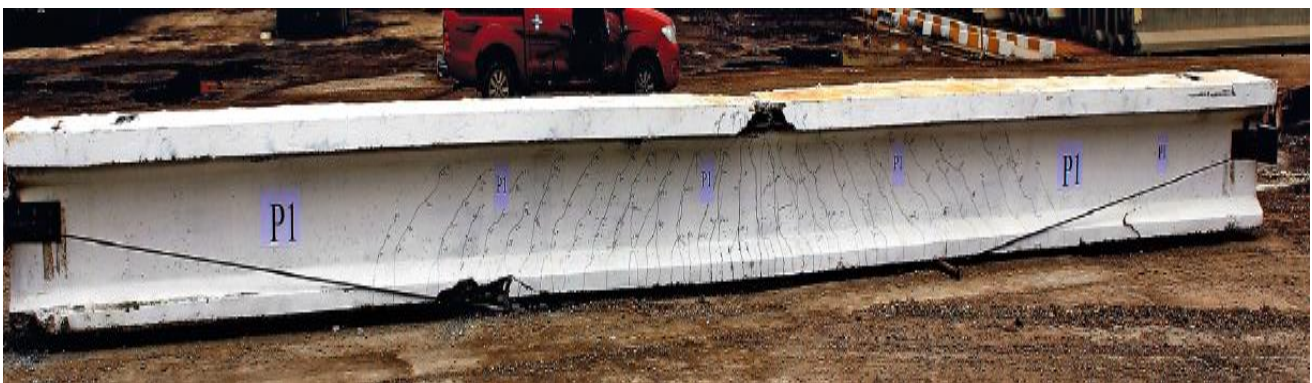
Figure 3. The crack pattern of PSC beam strengthening by external post-tensioning method [19]
