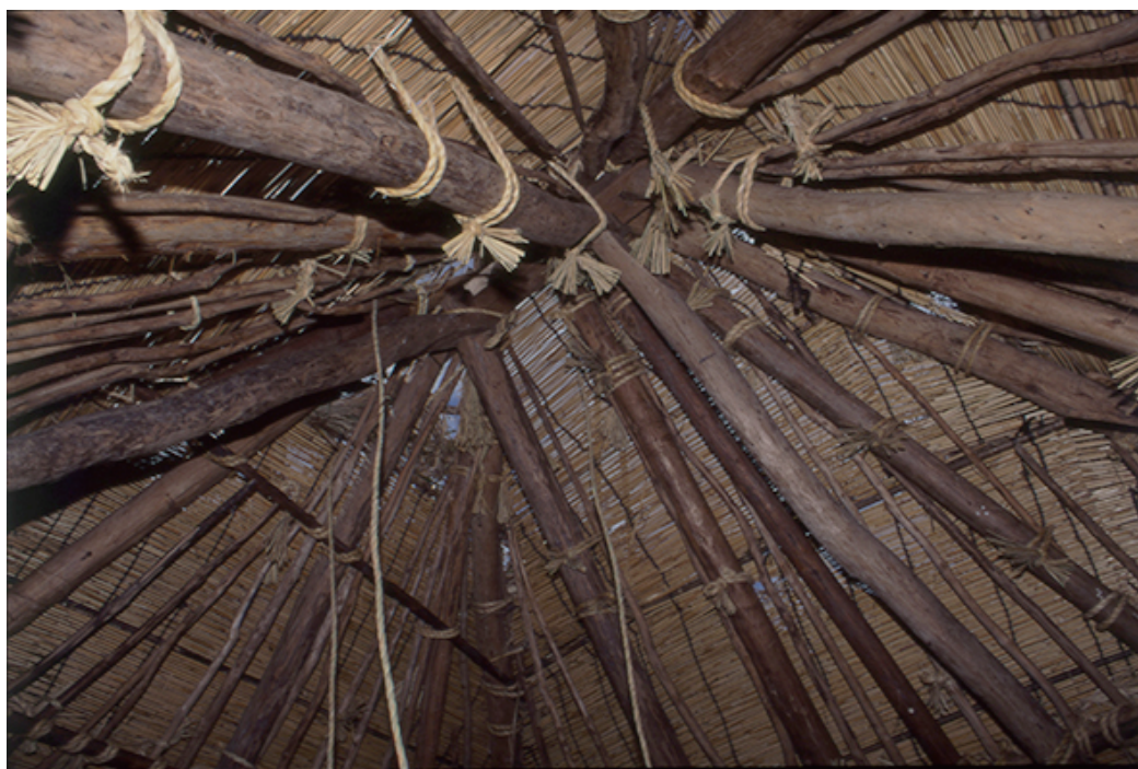
FIGURE 22. The rethatching work on Takakura storehouse is very rarely practiced now, March 1995.
