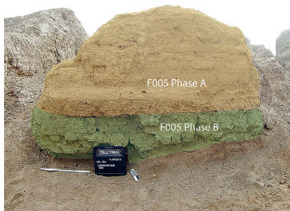
FIG. 12. Exterior of the western wall of the Q13-1 structure (Q13-1 F005). English bond is used in the upper level (Phase A) and Flemish bond in the lower level (Phase B).
