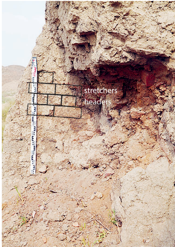
FIG. 13. Exterior wall of the L14 structure with bricks laid in the English bond pattern, looking west.
