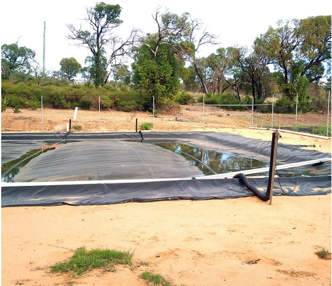
Figure 6. Photograph of the covered anaerobic digestion pond at Medina Research Station (photographed by Ayre).
