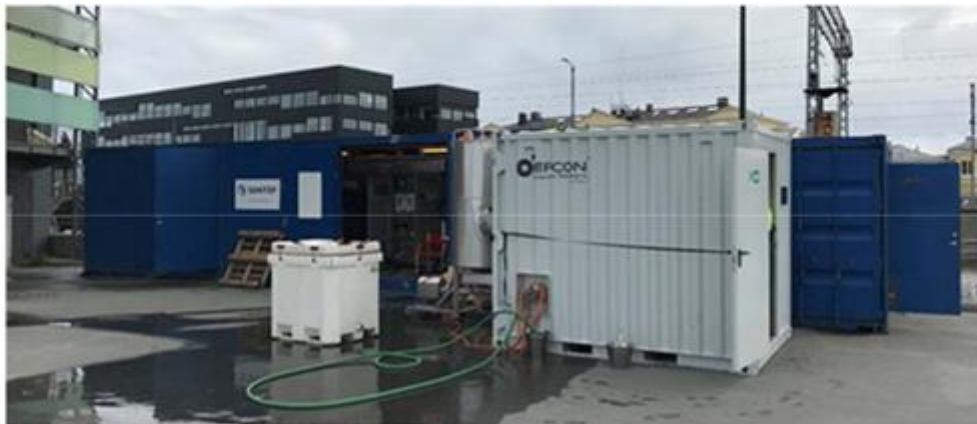
Figure 2: Containers with process line (left), evaporator (right) and steam generator (blue container behind the evaporator)
