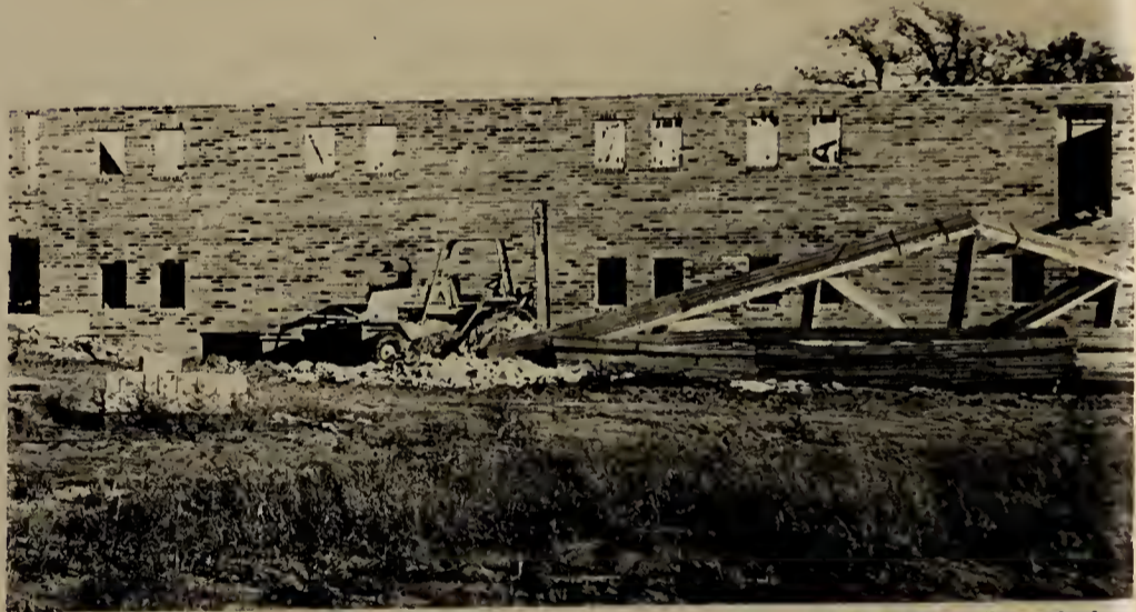
Brick wall rises for new Village Green Baptist Church, which is three-quarters of a mile north of campus on west side of Lambert Road. —Photo by Bill Bork.
