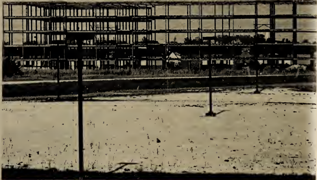
Steel girders shape new Raintree development along northern border of C/D property to Park Boulevard. It is a $35 million project. —Photo by Bill Bork.
