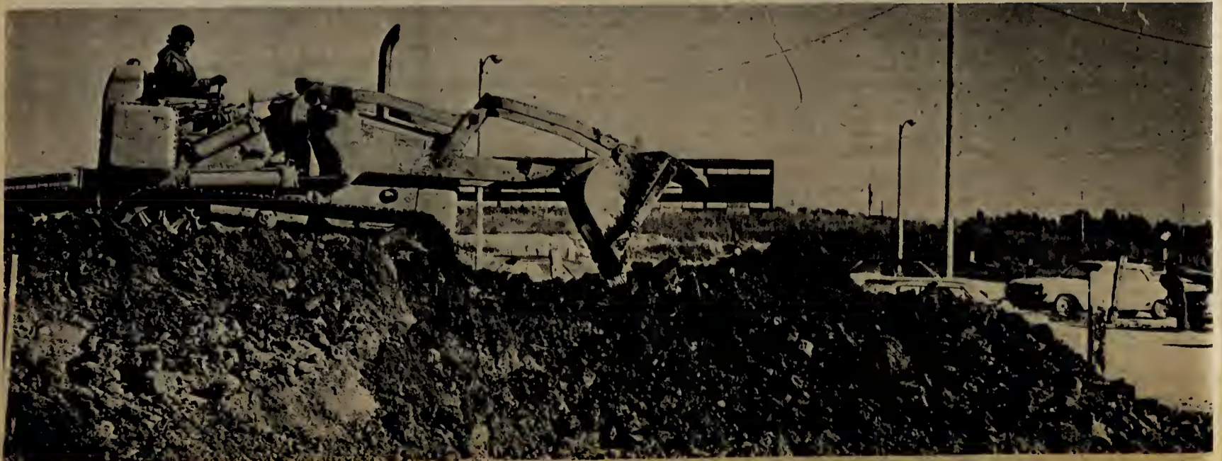
Tractor digs sewer line on easement along Lambert Road. Gravel parking lot is at right.
