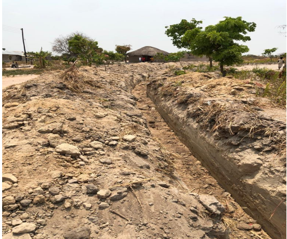
Both photos are showing works under way by a private actor in Mansa working on a Water Supply Project to the Peri-Urban areas in Mansa-Zambia, 2020.
