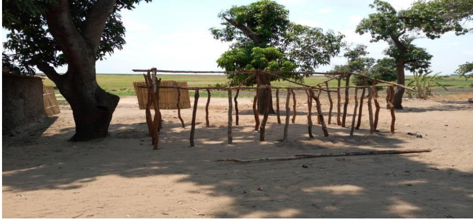
This is a house in making – Young man aged 23 years old was building “his house” on the day of the visitation. This picture (sticks) shows the structure – wall and roof
