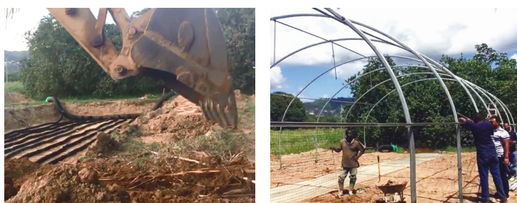
Installing underground pipes for cooling air and building the frame for the GIFT tropical greenhouse. (Photos: UWI & CARDI)
