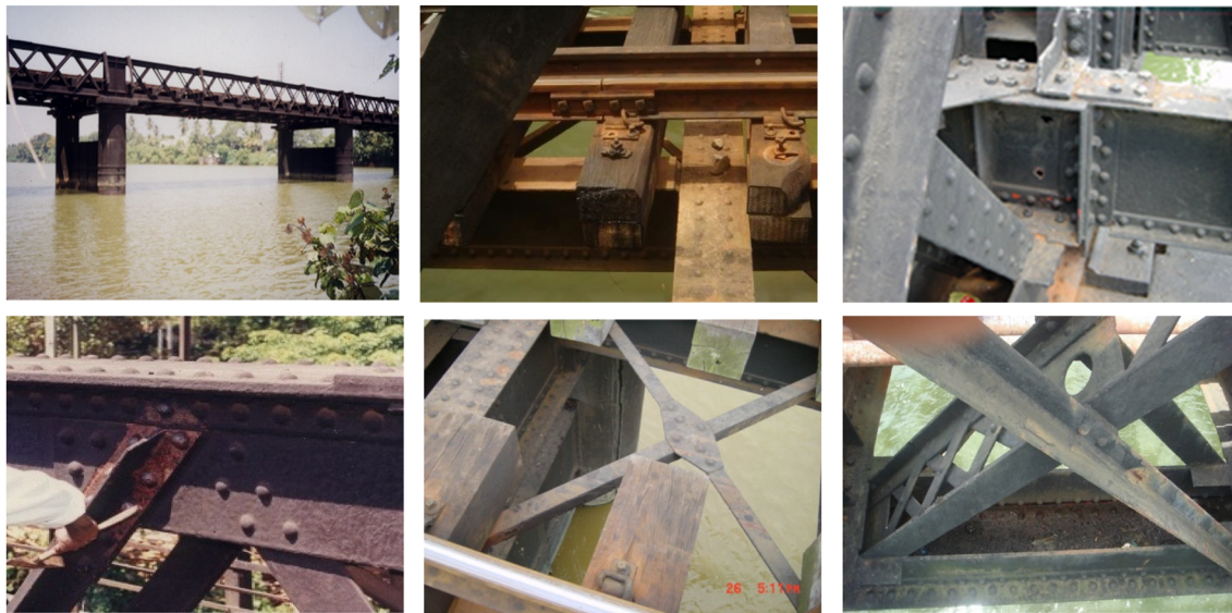
FIGURE 6 General view and some of the corroded locations of the bridge 4 [Colour figure can be viewed at wileyonlinelibrary.com]
