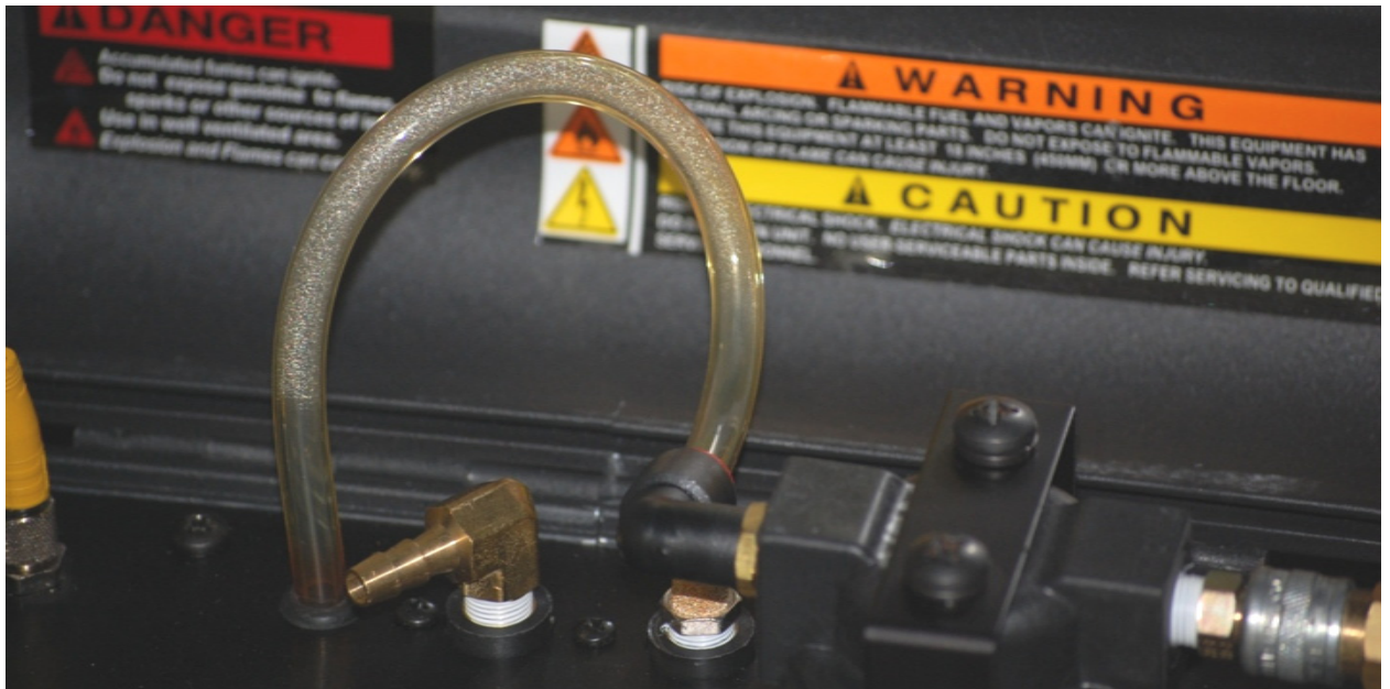
Condensation in the line coming out of the first inline filter
