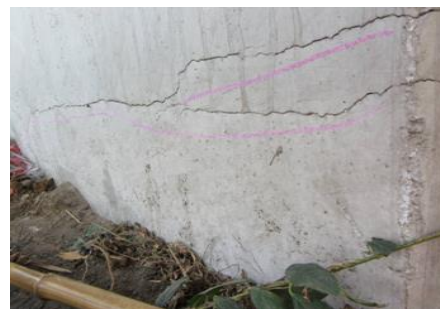
Fig. 5 – Bridge pier cracks
