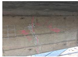
Vertical cracks in side span
