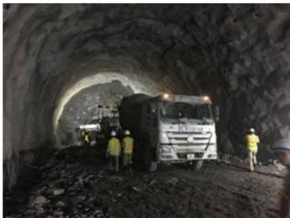
Fig. 30 - Drilling and blasting works when expansion the auxiliary tunnel in Hai Van project
