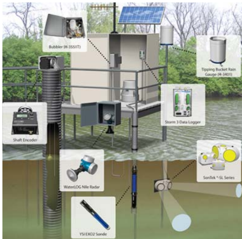
Fig. 4. WSNs node installed at the river side to detect water pollution
