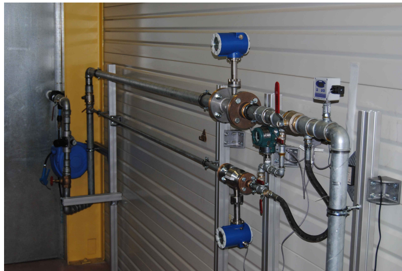
Figure 2.5: Compressed air regulation and quantification circuit.
