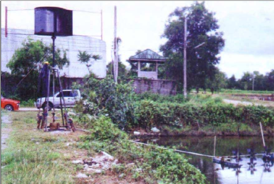
Fig. 6.42 Illustrates the completed set of the combined wind turbine at the selected shrimp farm
