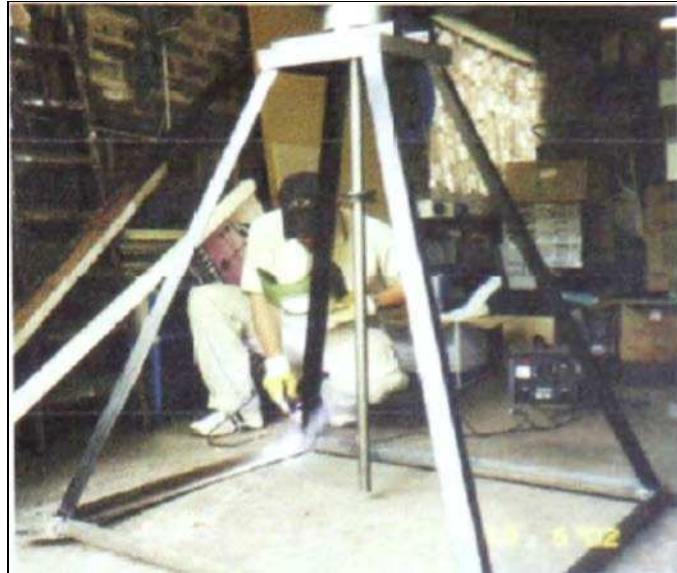
Fig. 6.6 Welding process to construct the tower and the base of the prototype
