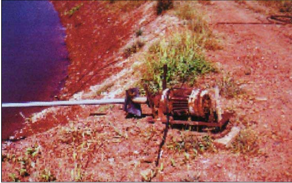
Fig. 6.34 Electrical motor used for water treatment in shrimp farm
