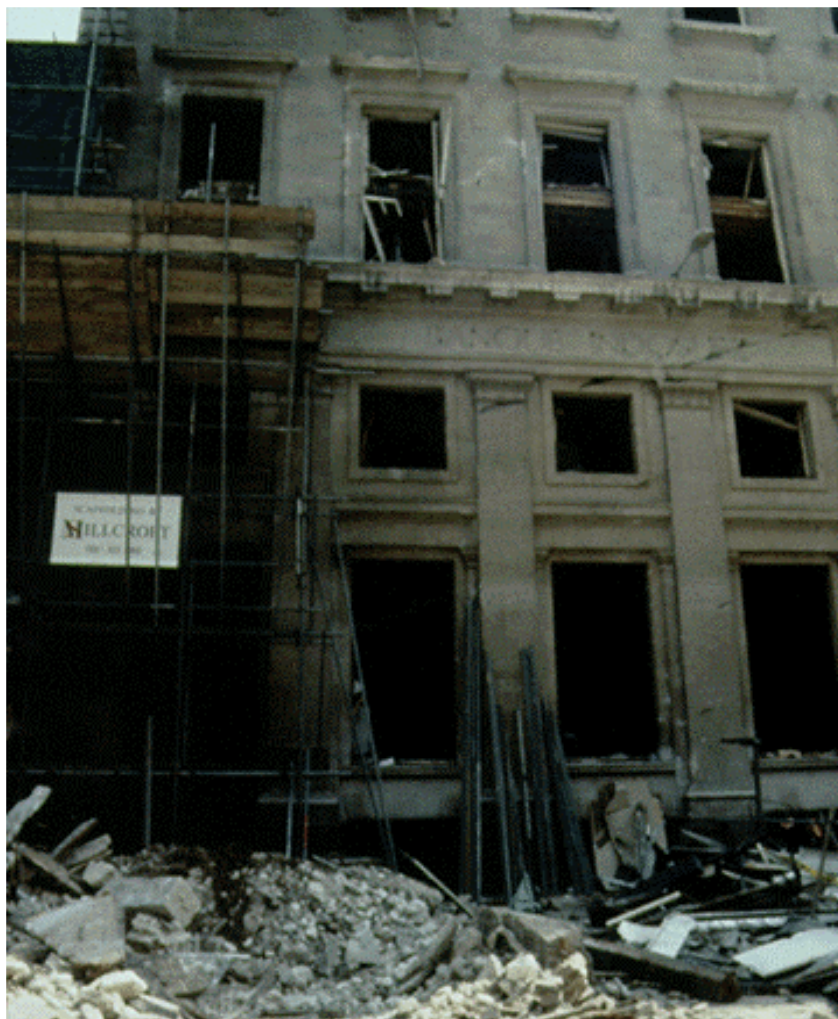
Figure 1. Damage to annealed glass windows in Bishopsgate
