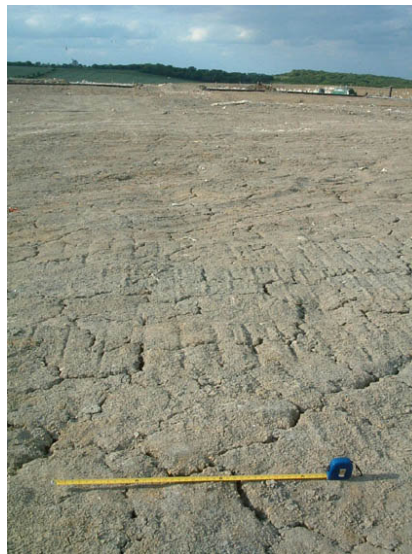
Figure 3-7. Brogborough landfill. A capped area. In this particular picture, the engineered Oxford clay presents visible cracks due to shrinkage of the soil. A one-meter length is shown in the image. (13 th June 2006).
