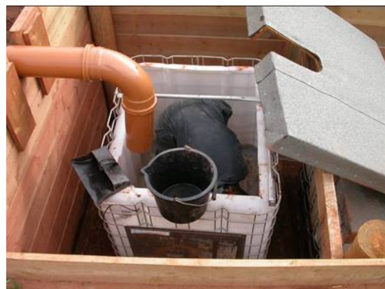
Plate 2.1-8 Inflow pipe, collection tank and tank lid
