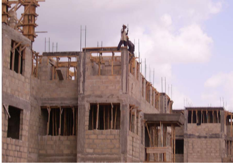
Picture 7.3 Site where PPE were not provided
