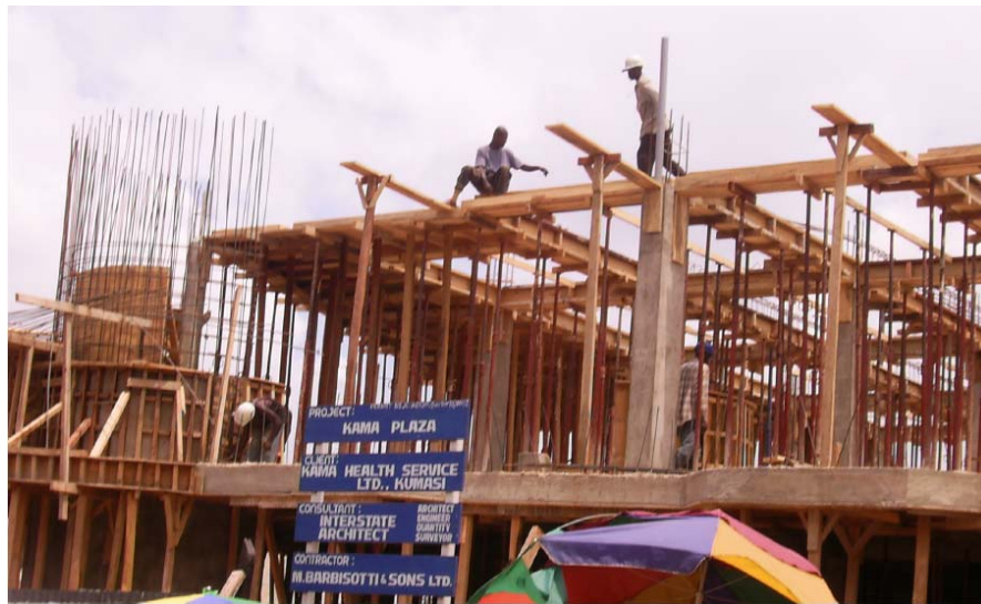
Picture 7.5 Non-use of PPE by some workers
