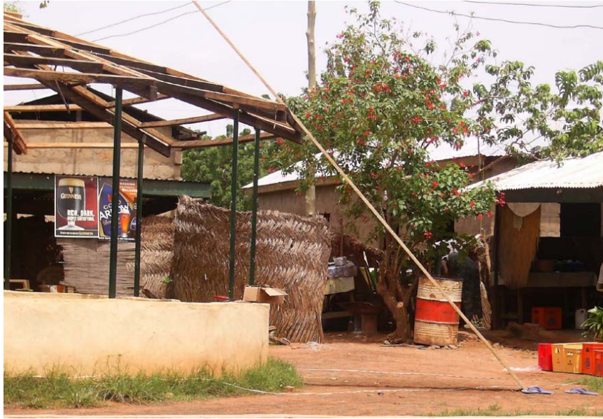
Picture 7.1 A plank used as a ladder to access roof
