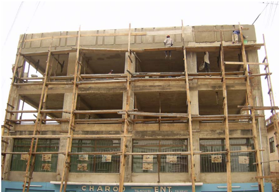
Picture 7.2 Insecure scaffolding used by plasterers
