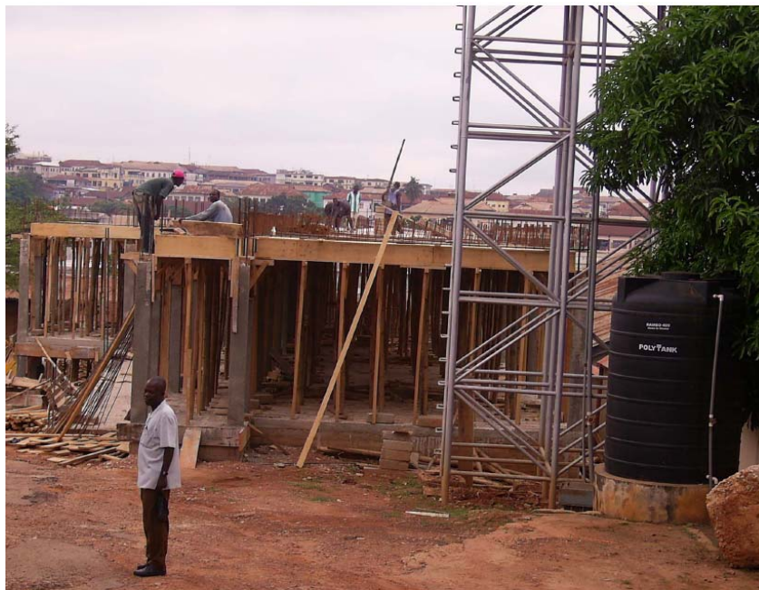
Picture 7.4 Workers working at a site where PPE were not provided
