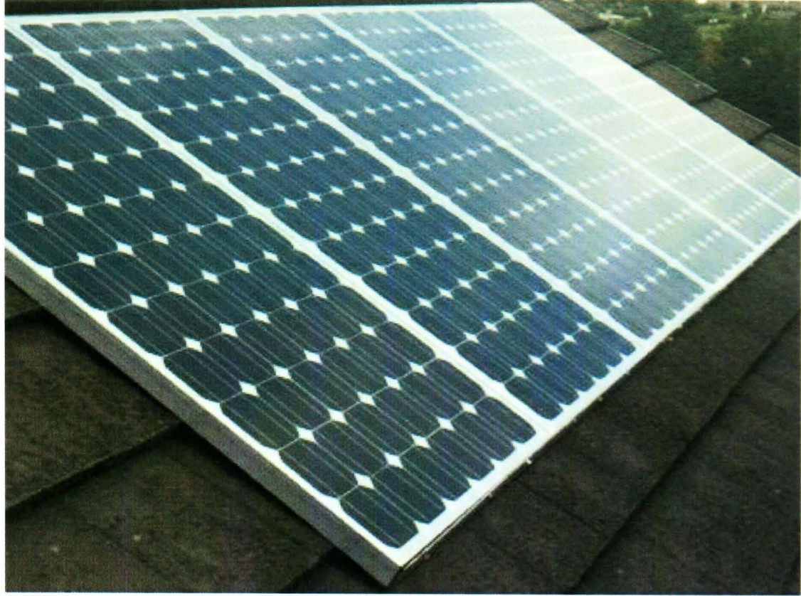
Figure 5.3 Example of ‘sun-in-a-box’ system on roof
