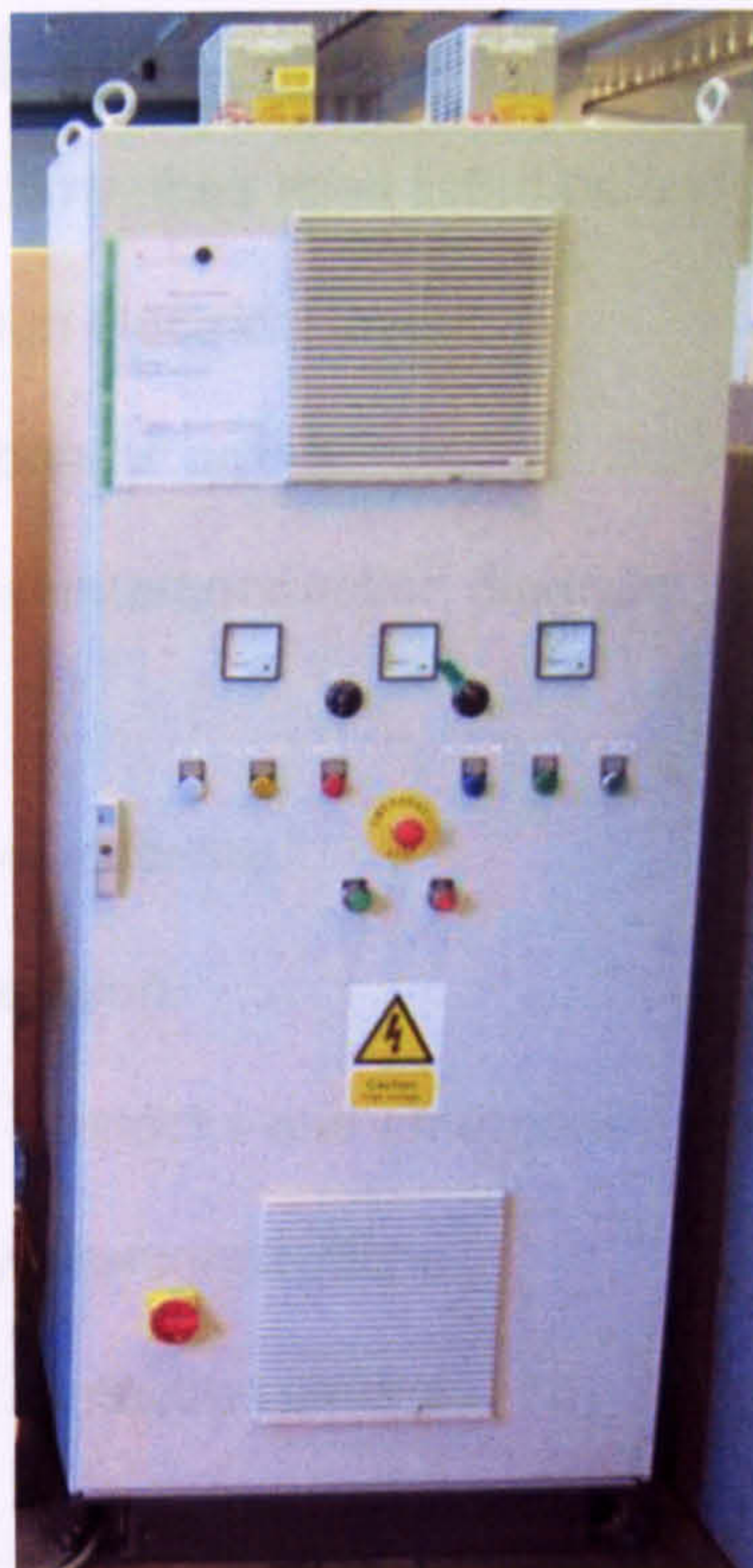
Figure D.31. DFIG control cabinet external photo.
