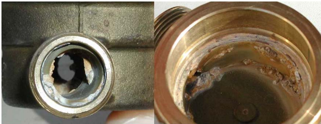
Figure 1-10 Limescale build-up in the inside of a single jet meter (Arregui et al. , 2005).
