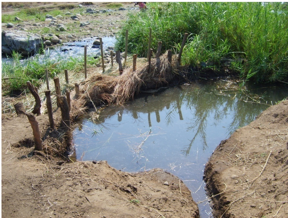
Fig. 5.3: A temporary dam formed by blocking a small stream. A diversion canal can be seen at the bottom right of the picture. The structure may wash away in the next rainy season.
