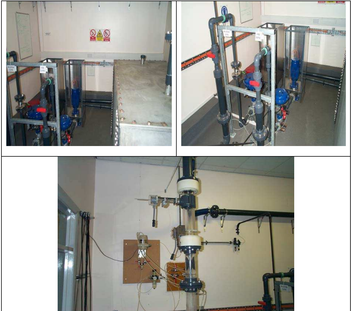
Figure 25. The oil-water loop. The tank and the pumps (top-left), the pumps the valves and the turbine meters (top-right), and the working section (bottom).
