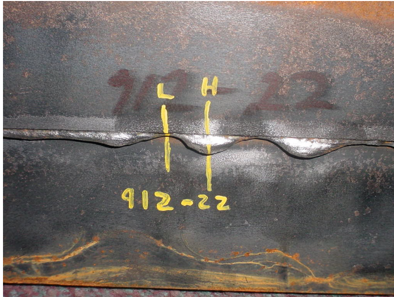
Figure 5.4 Typical Bead Humping Defect in a Lap-Fillet Weld
