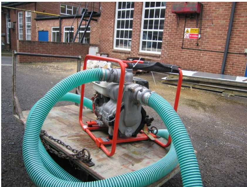
Figure 41: Pump unit and connection hose
