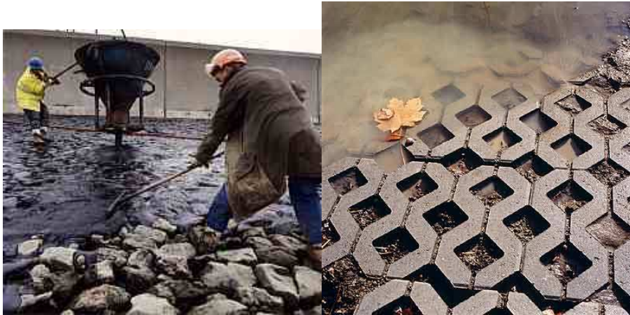
Figure 5 Showing stone pitching being bonded by asphalt and an interlocking concrete block system
