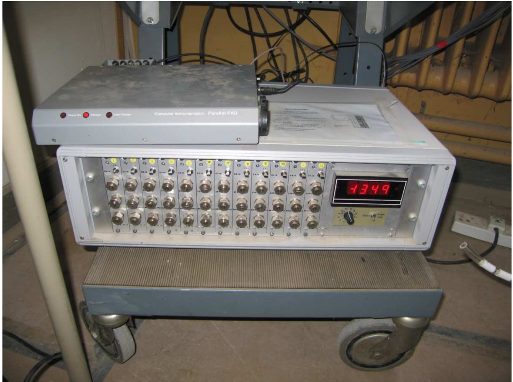
Figure 40: View on bridge amplifier and ‘Pad’ data logger
