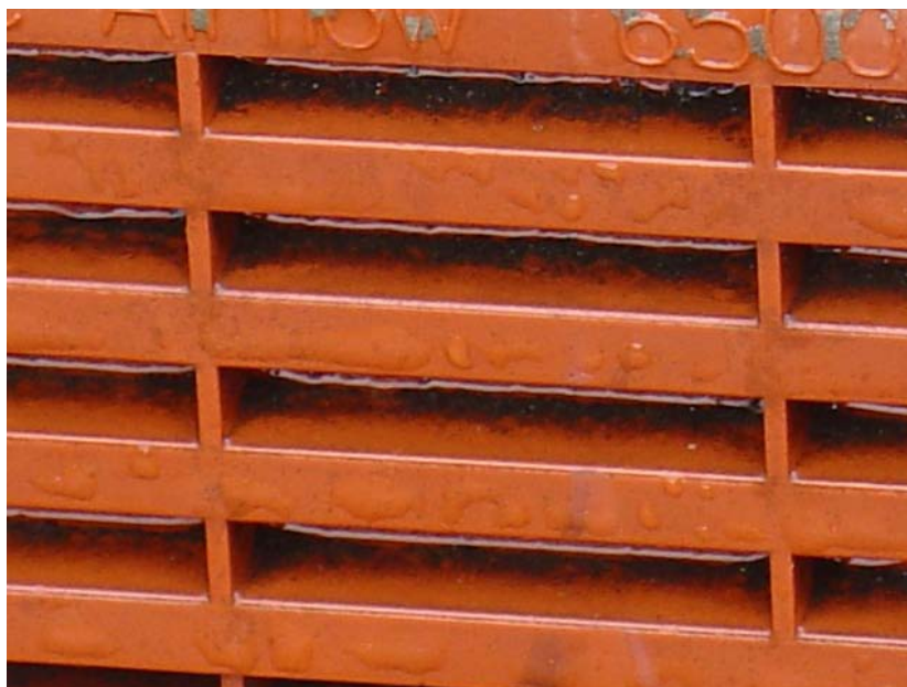
Figure 6-19 The wall vent in the playground - School A
