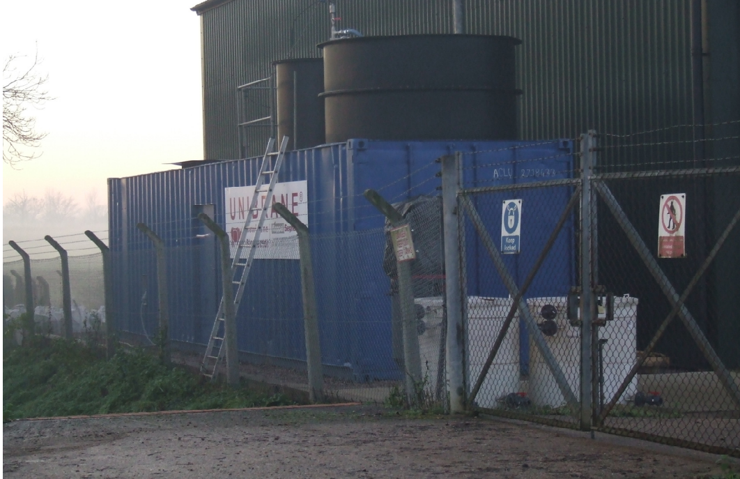
Figure 4-8 – The containerised pilot plant showing the tops of the membrane and aeration tanks.
