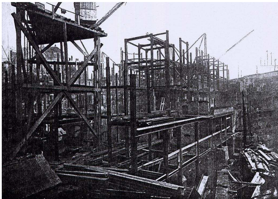
Figure 114 Milburn House under construction. (Jeans, H. [1926] Modern Building . London: Edward J. Burrow & Co. for Stephen Easten Ltd).
