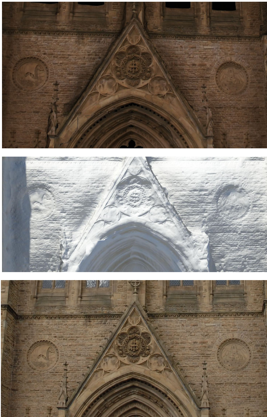
Figure 6.17: Close up view of an interesting area of the façade. (Top) Relit model. (Middle) Recovered geometry. (Bottom) Photograph of the same section.
