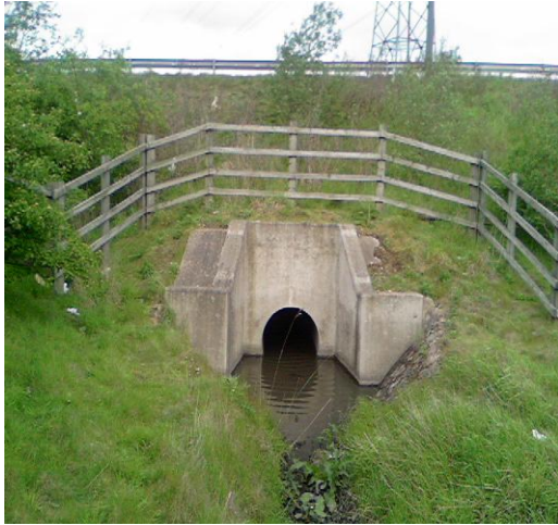
Photo 4.1 1 st sample point. Inlet into the treatment system with the A50 above.
