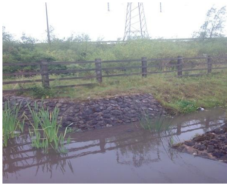
Flooded ditch linking motorway runoff to the inlet to the separator was flooded
