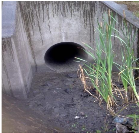
Inlet prior to the storm
