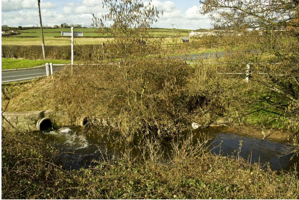
Photo 4.10 Final effluent of the Osgathorpe sewage works
