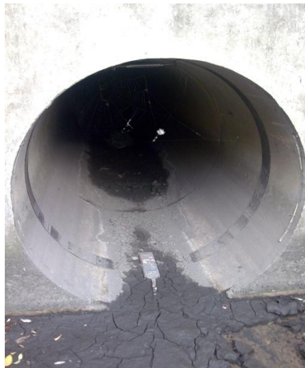
Photo 4.7 Flow meter in the inlet during dry weather period
