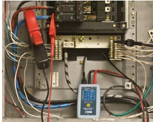
Figure 8.4: A Chauvin Arnoux data logger recording energy data off a load centre
