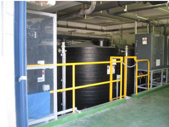
Figures 3.4.2 and 3.4.3 Storage tanks for H 2 SiF 6 and safety monitoring equipment
