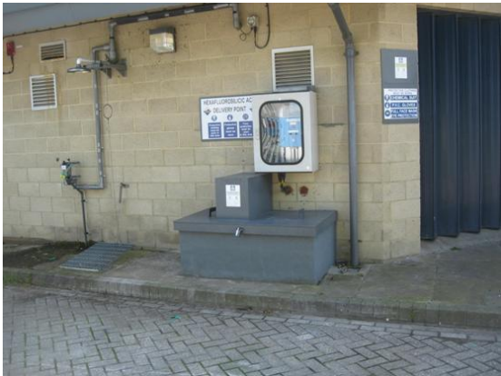
Figure 3.4.1 Storage area H 2 SiF 6 water treatment works
