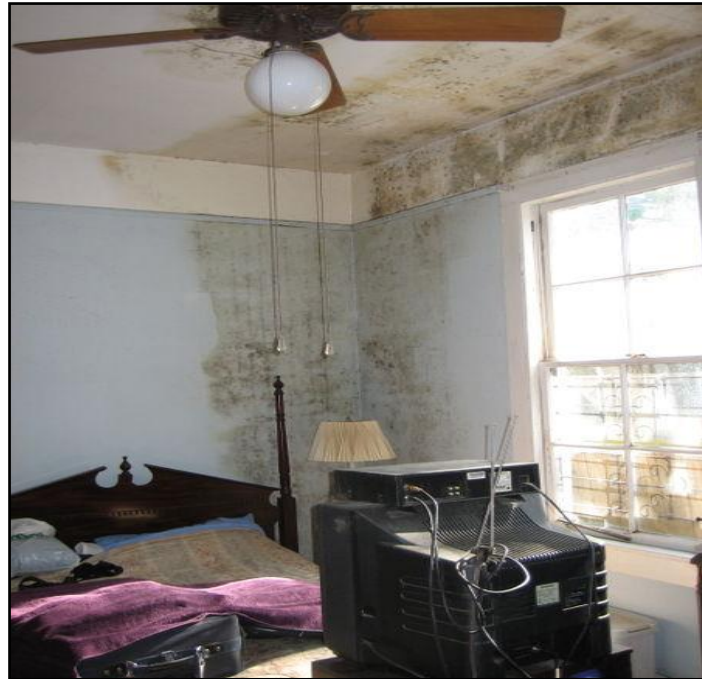
Plate 1.4 Mould affected home
