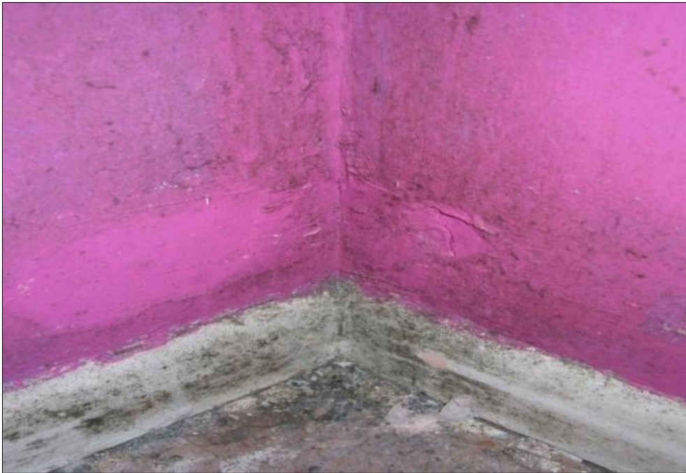
Plate 3.1 Fungal growth on bedroom wall and skirting board, Marsh Farm, Luton
