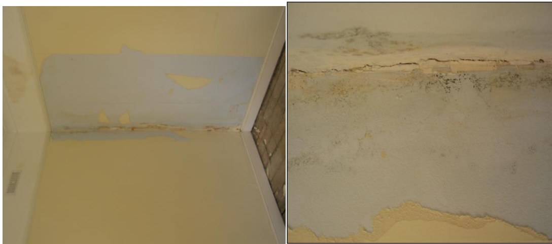
Plate 3.5 Visible fungal growth on the ceiling and wall, Cricklewood
