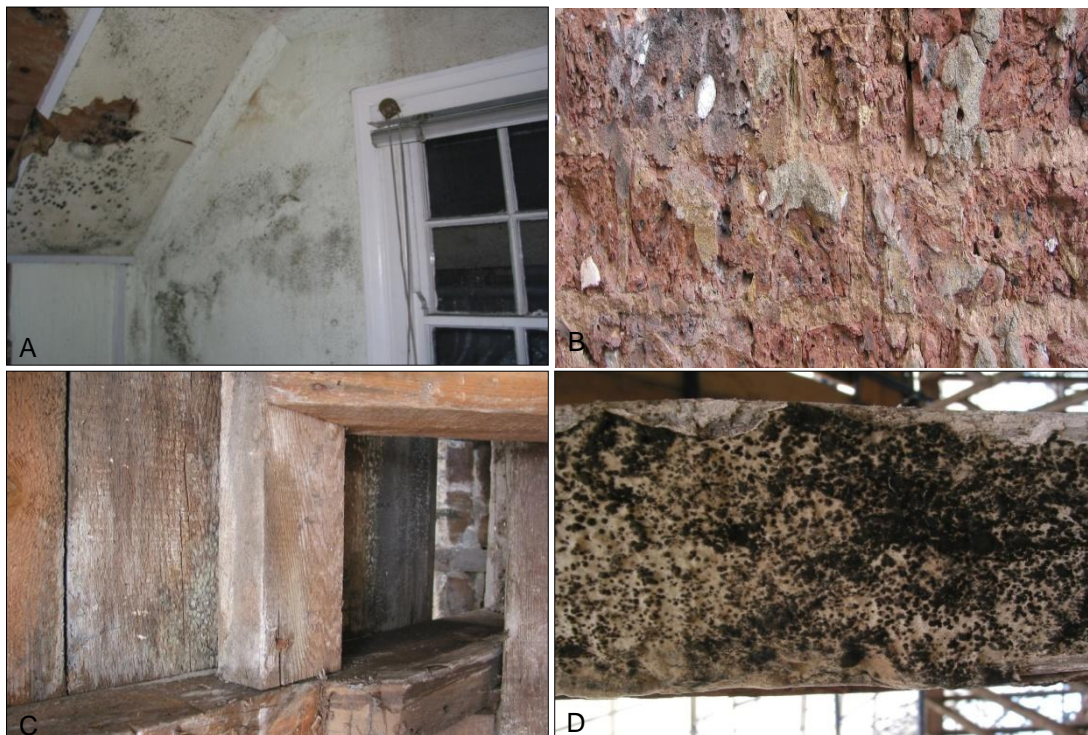
Plate 3.6 Visual fungal growth observed in the Victorian stable block, Watford (A) Room 1, east and north facing walls (B) Room 1, south facing brickwork (C) Room 2 clocktower frame, (D) Room 2, wooden roof member with plaster.
