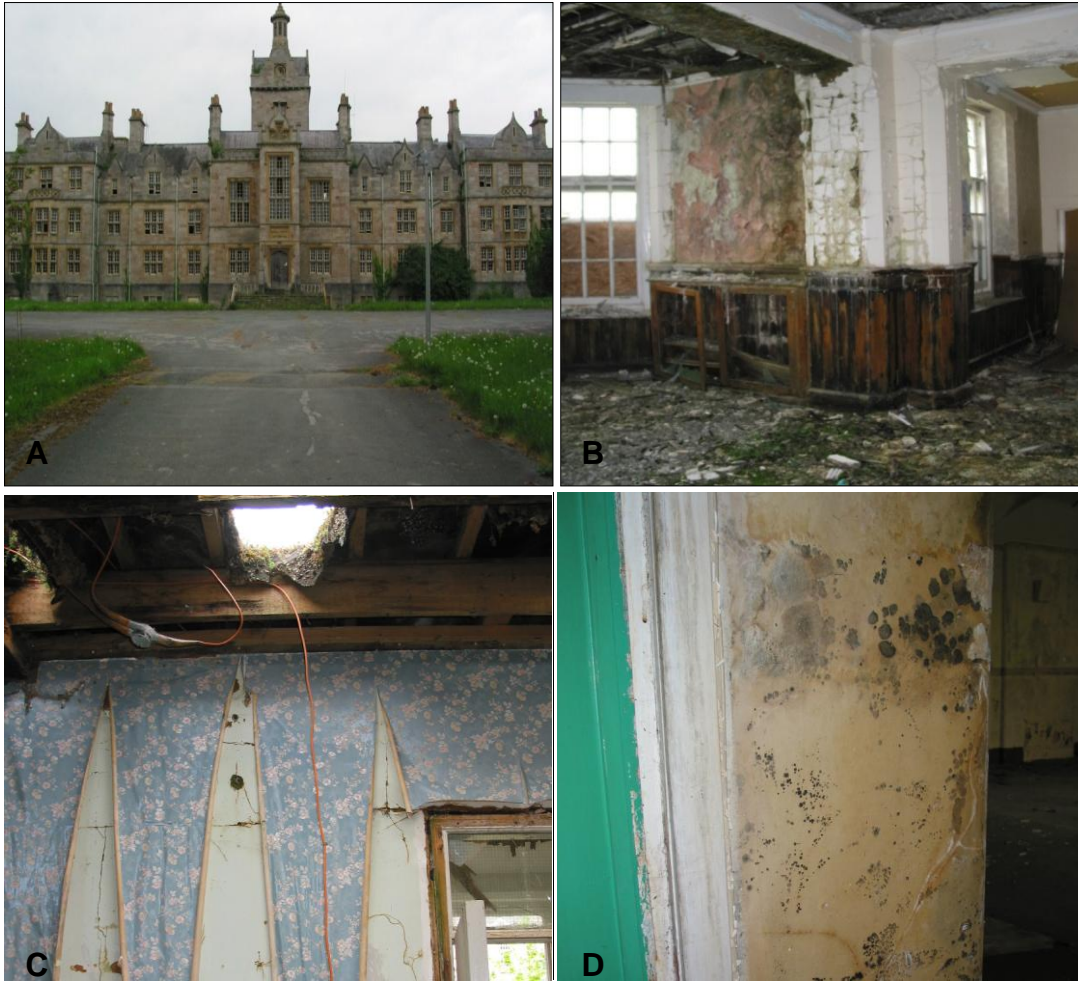
Plate 3.8 (A) Entrance to building 1, (B) Severely infested room in building 1 (C) water damaged room in building 2 (D) infested wall in building 2, Denbigh Hospital, north Wales
