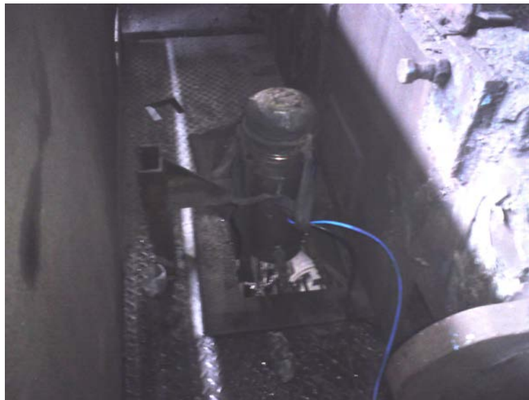
Figure 5.6 : Installed camera enclosure
