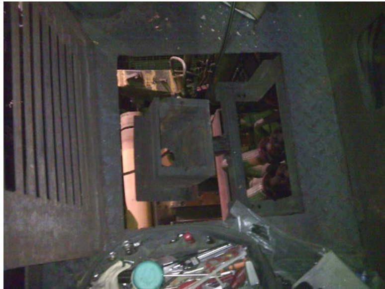
Figure 5.5: Hatch and pre-existing mounting bracket
