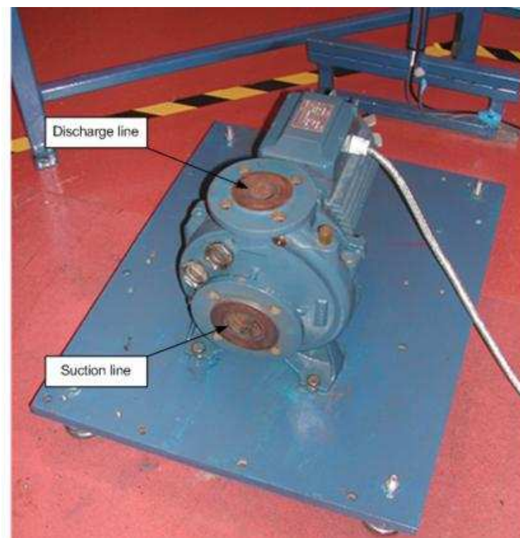
Figure 4-1 Pump secured to floor
