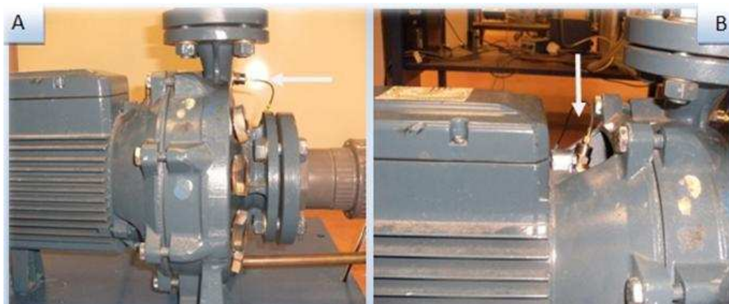
Figure 4-12 Positions of the accelerometers (a)- At outlet of the pump (b) - Between pump casing and motor of the pump
